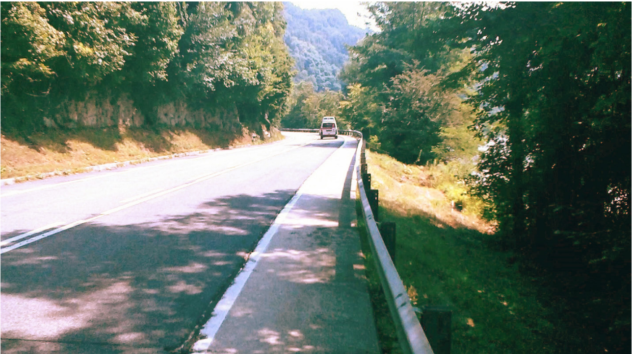
Paved shoulder on road number 3 between Grein and Hirschenau (daily section 17) – too narrow for safe cycling outside built-up area, effective width further reduced by safety barrier.
